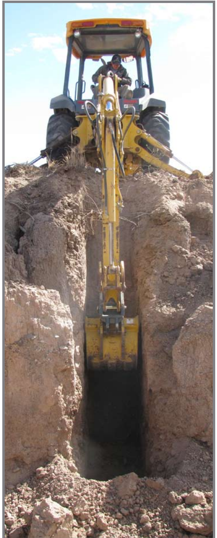
Lance Jarratt volunteers his time and backhoe to cut essential exploratory trenches that enable CBBS archaeologists to interpret and document natural and cultural soil strata at the site. Photo by Andy Cloud.
