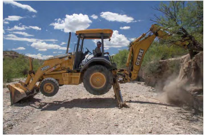
At the Deep End site, heavy machinery was employed to excavate several deep trenches and expose buried Late Archaic deposits. Photo by Samuel Cason.
