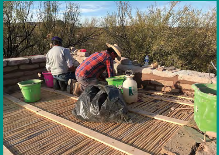
Louis Madrid (left) and Rosalio Sanchez mortaring in new parapet adobes. Photo by David Keller.
